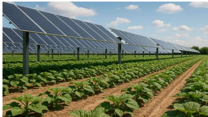
Fig. 2: An agrivoltaics system showing elevated PV panels above crop rows
